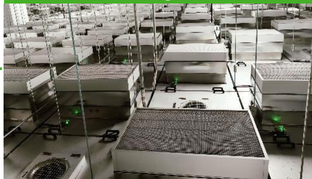
3. Cleanroom ceiling from above
