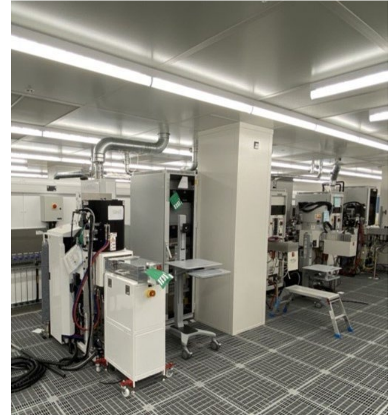
Systems installed in university labs
